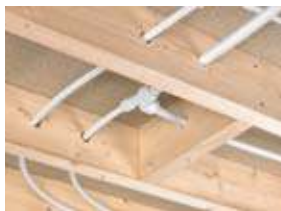
Easy cabling. Fewer joints
